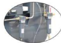
Pre Filter and After Filter
